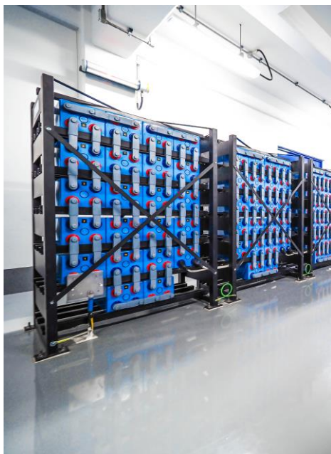
LITHIUM BATTERY LEAKS
